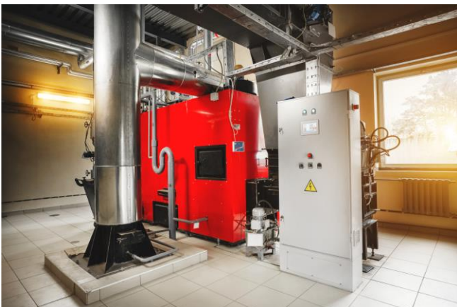
Wood Chip Boiler
