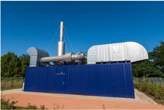
Combined Heat and Power Plant Container
