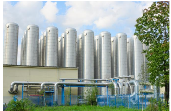
Large-scale Thermal Storage
