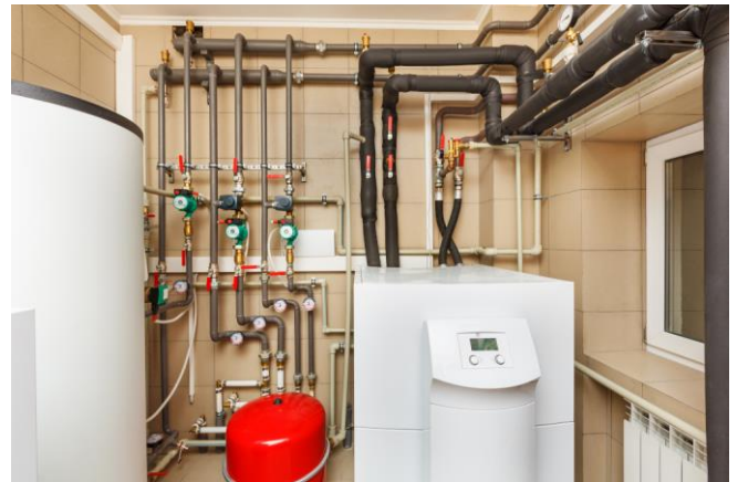
Apartment based / decentralised heating
