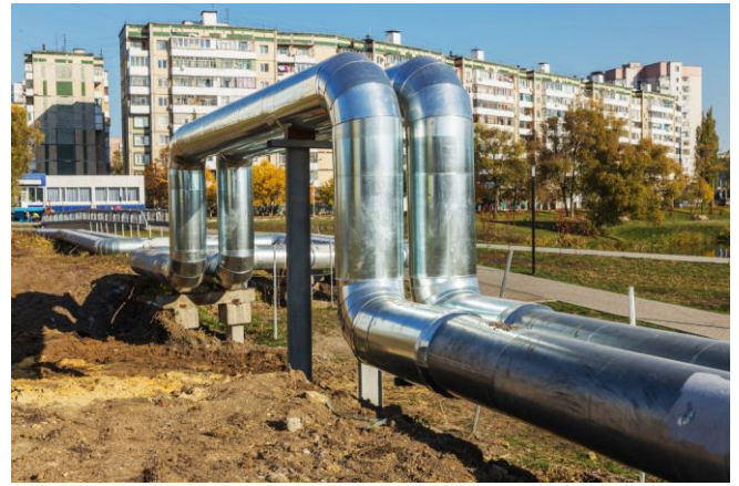
Centralised heating infrastructure
