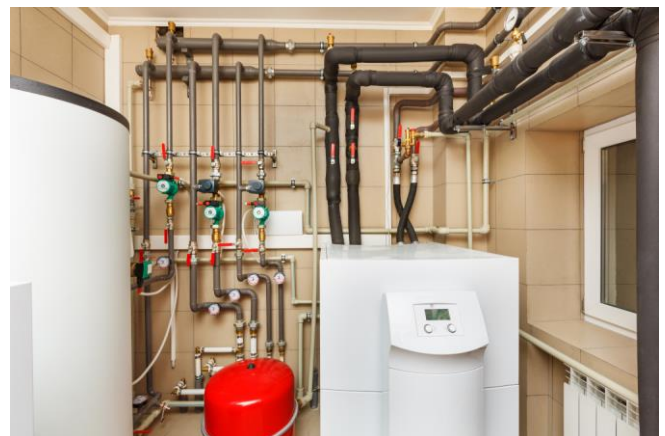
Medium-sized Electric Boiler
